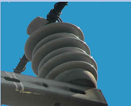
LP Insulator Crack
