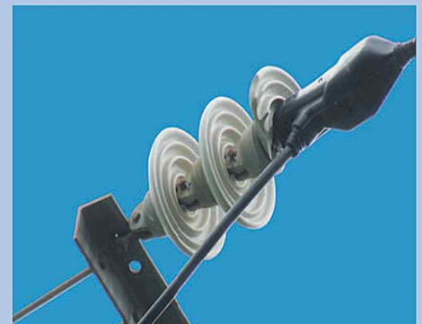
Suspension Insulator Broken
